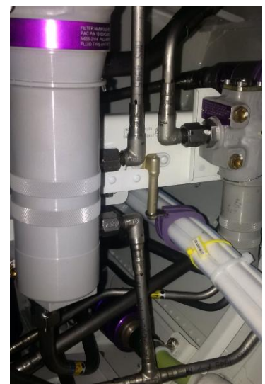
AC 20636 & Subs Supporting Hardware Configuration
