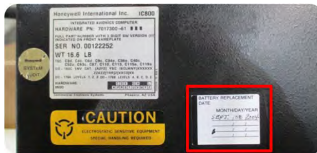
Figure 1 - Battery replacement label Location
